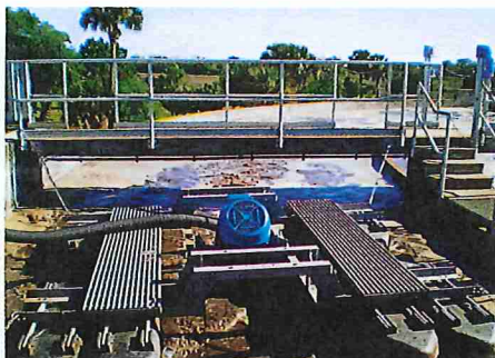
The aerator and mixers provide dual functionality, which can save on operating and energy costs.
