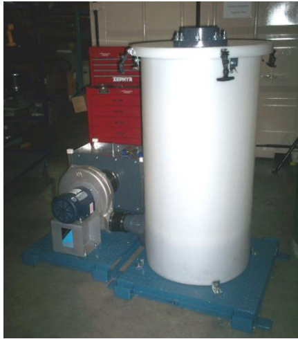
Quebec Sewage Pumping Station
